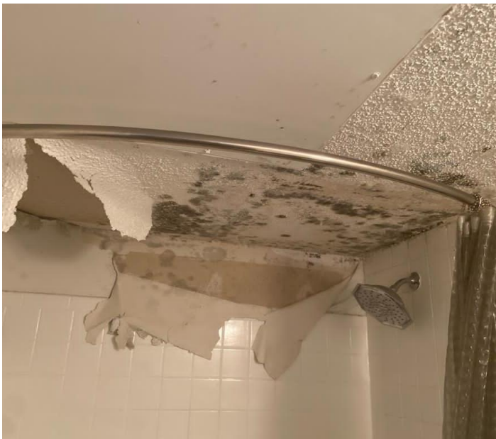
Figure 1: Neglected ceiling leak causes mold in bathroom. Image: BASTA
